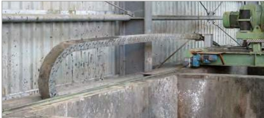
Steel cable carriers with steel band cover on a shredding system Photographs: Lindenschmidt KG
