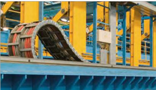
Steel cable carriers on a laser cutting machine Photographs: Meyer Werft GmbH
