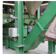
■ Scraper conveyor under a hopper system for aluminum chips
