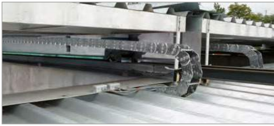
Steel cable carriers on a movable roof construction Photographs: Lindenschmidt KG
